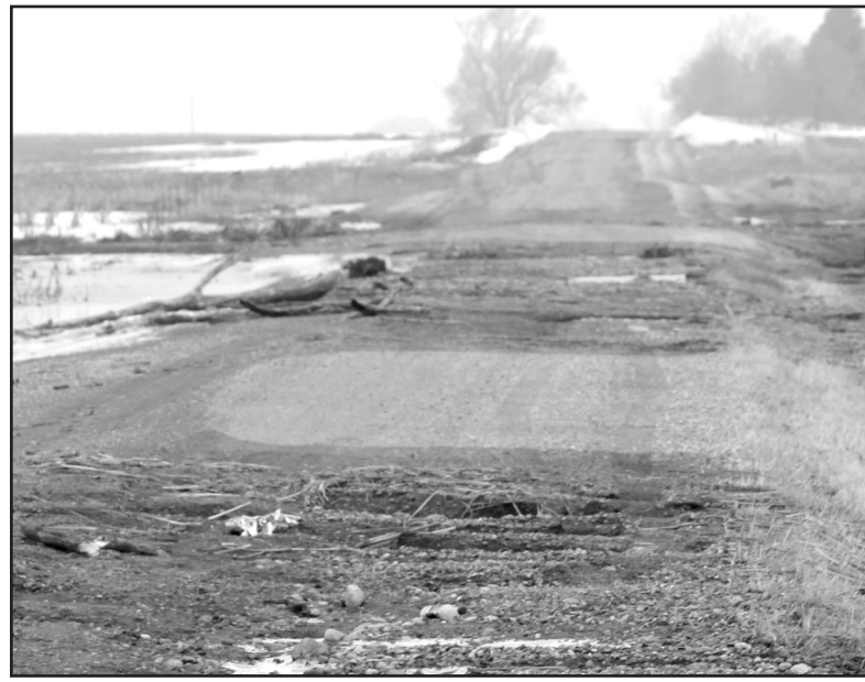
Damage to county roads from flooding that will need repair after the ground dries.
